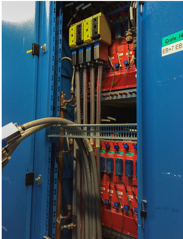
Figure B.2.4: P5 HV racks during the first installation of the Multiboxes in 2015
