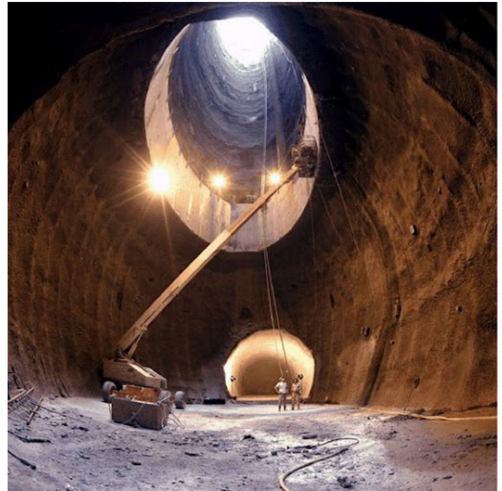
Shaft to the SSC tunnel di SSC, located at about 10 meters underground. The planned tunnel had a circumference of 87 km.
