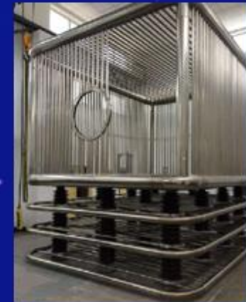
Accelerator tank installed in Aug. 2016
